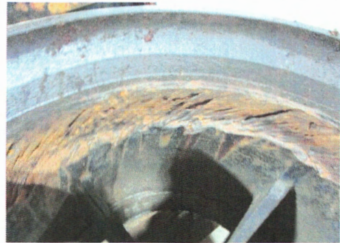
Extreme damage to bowl skirt where impeller runs
